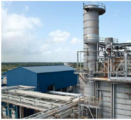
Energas Varadero's combined cycle generating facility produces lower GHG emissions for each gigawatt hour (GWh) of electricity than other facilities.
