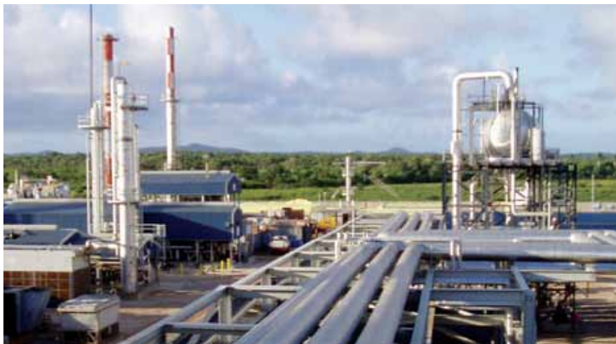
Energas S.A. power plant in Varadero, Cuba
