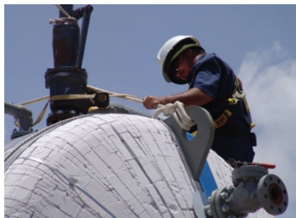
A Cuban worker is shown above, installing new equipment for Sherritt Power's Energas joint venture.
