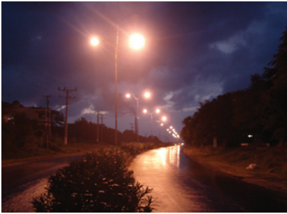
The photo above is an example of new street lighting provided by Sherritt in Cuba. This photo is taken in Boca de Jaruco, between Havana and Matanzas.
