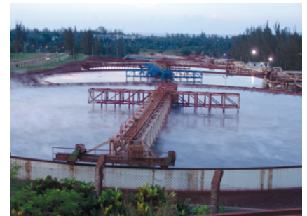
The counter current decantation (CCD) process at the Moa plant is a major user of water as the concentration of metal is increased in solution.
